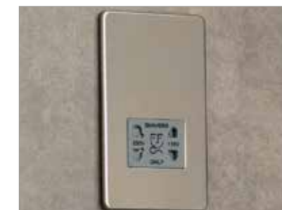
Ventilation/ Shaver Sockets 79
