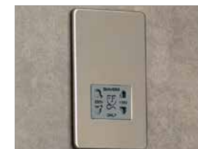
Ventilation/ Shaver Sockets 79
