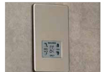
Ventilation/ Shaver Sockets 79
